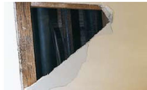
Asbestos insulating board (AIB)
