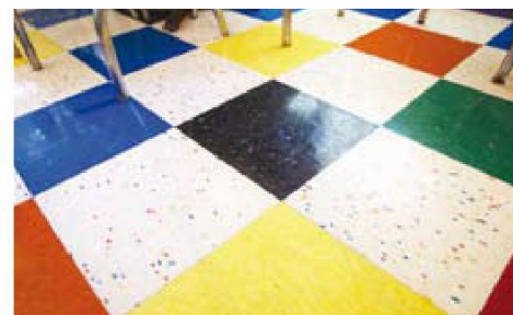
Asbestos-containing floor tiles
